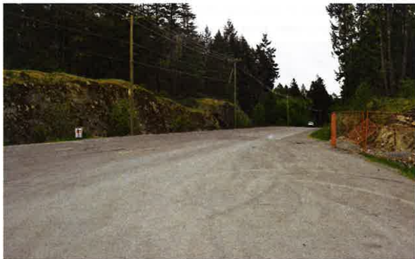
1: Willis Point Road & Hartland Access - Worn pavement markings
