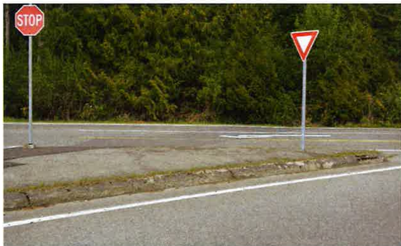
5: Willis Point Road & Wallace Drive - Damaged traffic island
