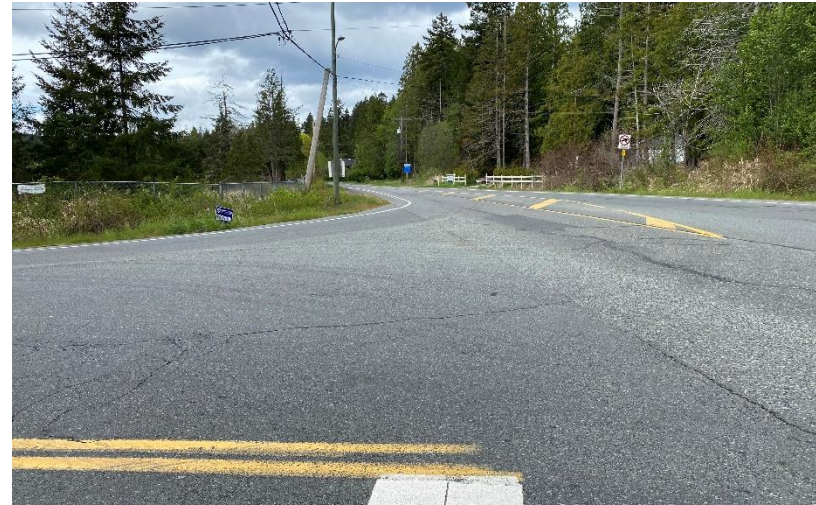
2: Willis Point Road - Looking north on Wallace Drive (reasonable visibility but could be improved by trimming vegetation)
