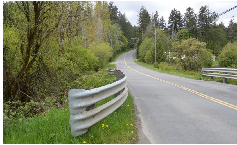
8: Hartland Avenue – Frequent horizontal and vertical profile changes. No shoulders.
